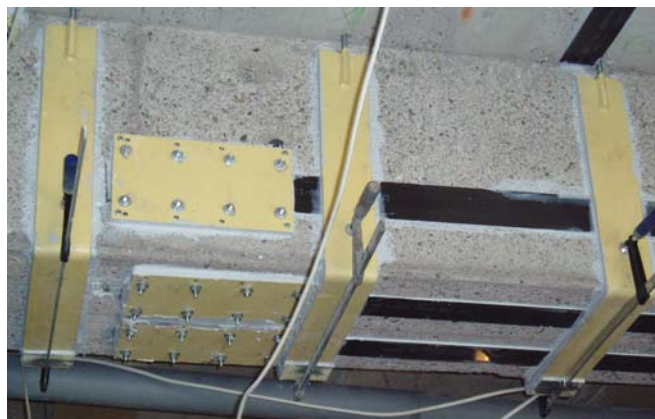
Fig. 14 Beam, strengthened with prestressed CFRP-strips and steel plate stirrups, anchored in the compression zone.
