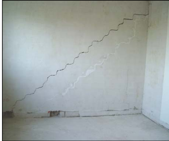
Fig. 11 Underdesign of concrete slab causes excessive slab deflection and wall cracks.
